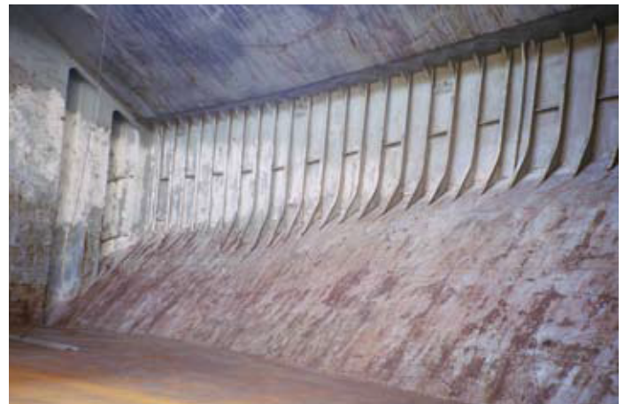
^ Loose rust and scale must be removed
