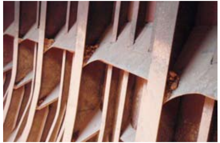
^ Residue of previous ore cargo caught in the frames
