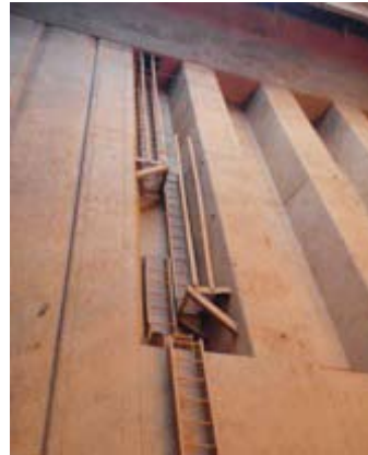
^ Hold ladders should be in good condition
